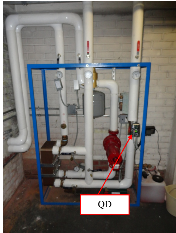
Dump Radiator HX and BTU Meter (QD)
