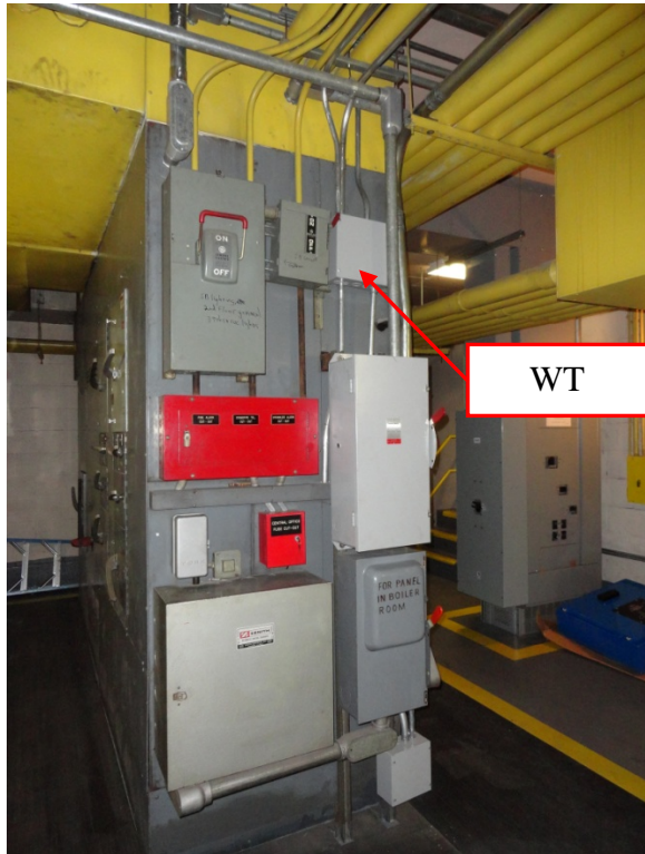
Building Main Switchgear
