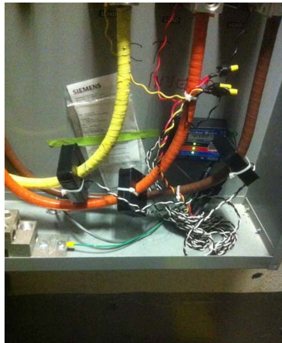
Newly installed Wattnode power meter.
