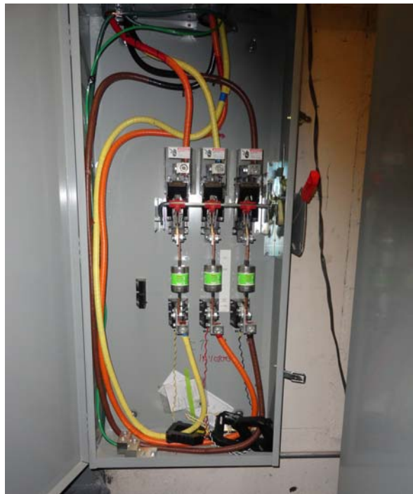
Initial Veris H8035 Power Meter, located in 480V switchgear.
