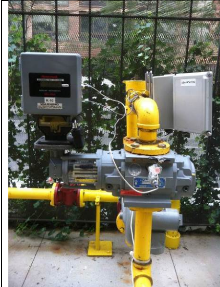
Roots gas meter (right) and Honeywell Mini-Max pulse module (left).
