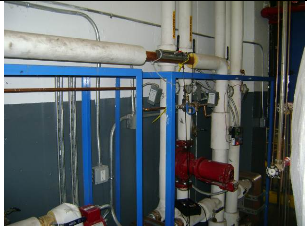
Recovered heat loop #1 flow (FL1) verification location.
