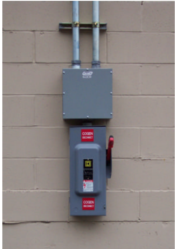
Ground-Level Disconnect at Rear of Store
