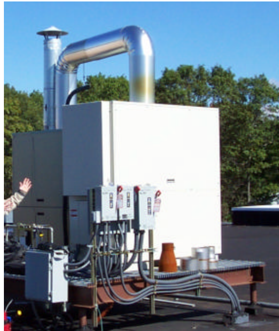
Microturbine with Disconnects at Roof
