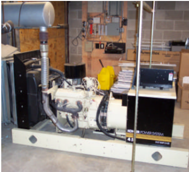
Standby Generator with Automatic Transfer Switch for Emergency Circuits
