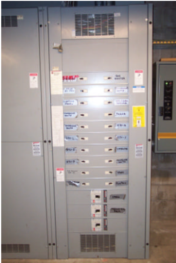
Store Main Distribution Panel (480/277V, 1600 amp)
