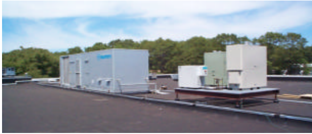
CHP Skid and Munters AHU (before Screens were installed around AHU)
