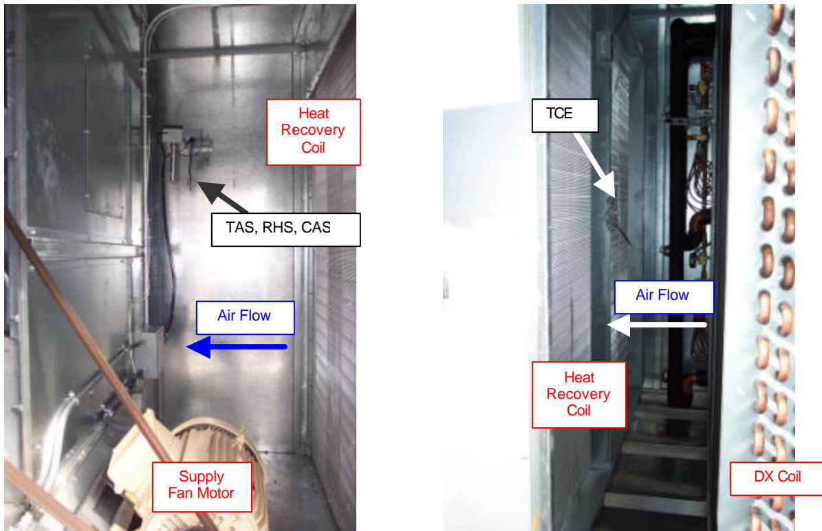
Figure F-15. Supply and Entering Heat Recovery Coil Sensors - Airflows Shown in Blue, Sensors in Black, Equipment in Red
