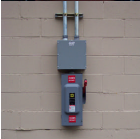
Ground Level Disconnect at Rear of Store
