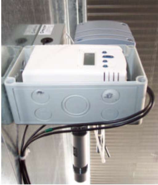
Figure F-16. Closeup of Supply Sensors
