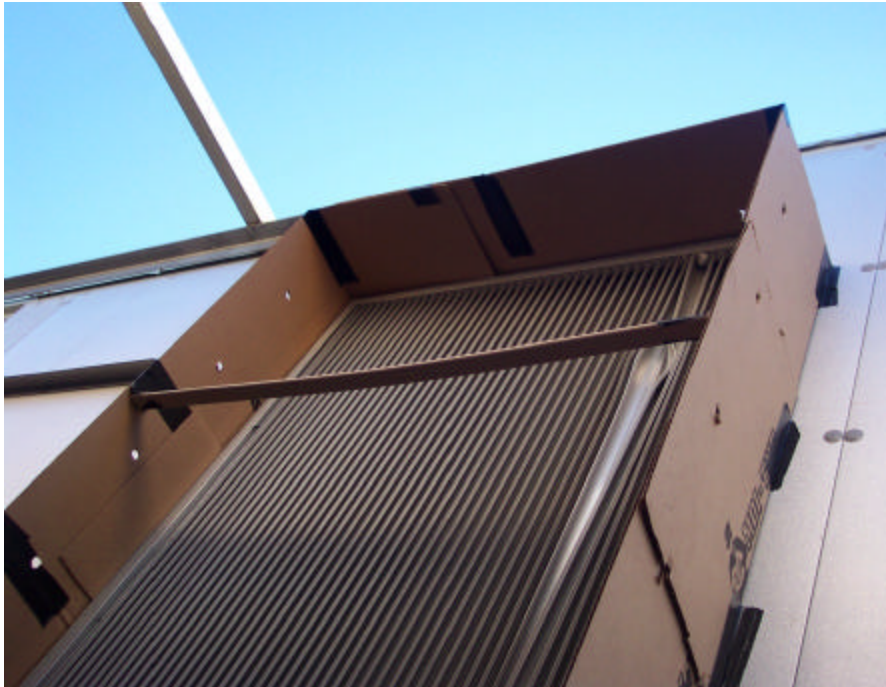
Figure F-22. Munters Fresh Air Intake with Cardboard “Duct” Added For Flow Measurement
