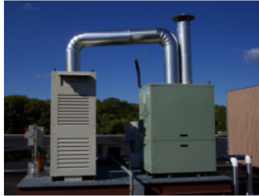
Finished Skid - Front
