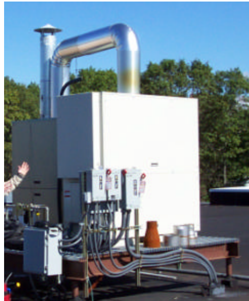
Microturbine with Disconnects at Roof
