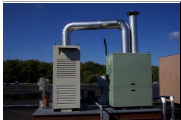
CHP Skid Located on Roof - Front
