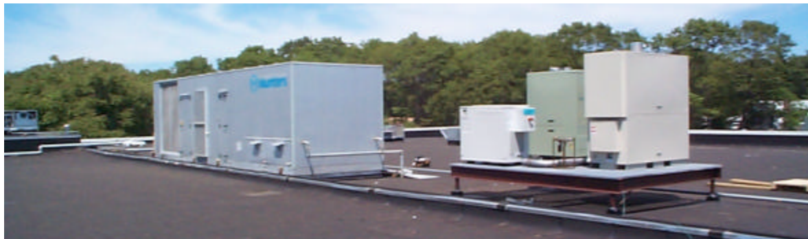
Figure 3. AHU and Microturbine Skid (During construction, before screens installed on Munters AHU)
